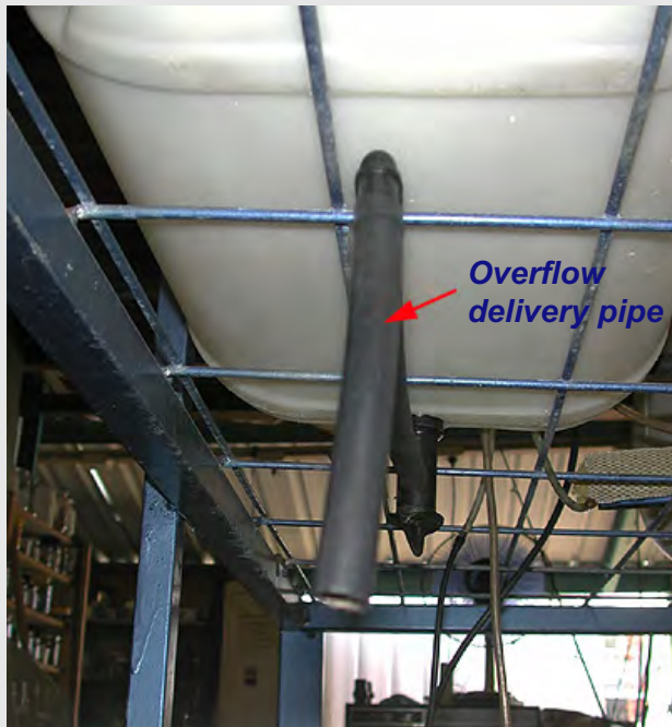
Individual tank on rack showing overflow delivery tube
